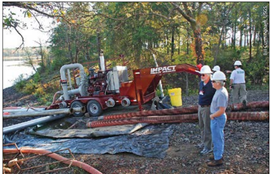
Pumping water from a lake for hydraulic fracturing in the Fayetteville Shale of Arkansas.
